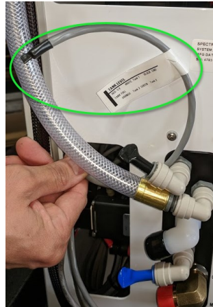
5 Conductor wire: Tank Full Switch, Green + Orange
